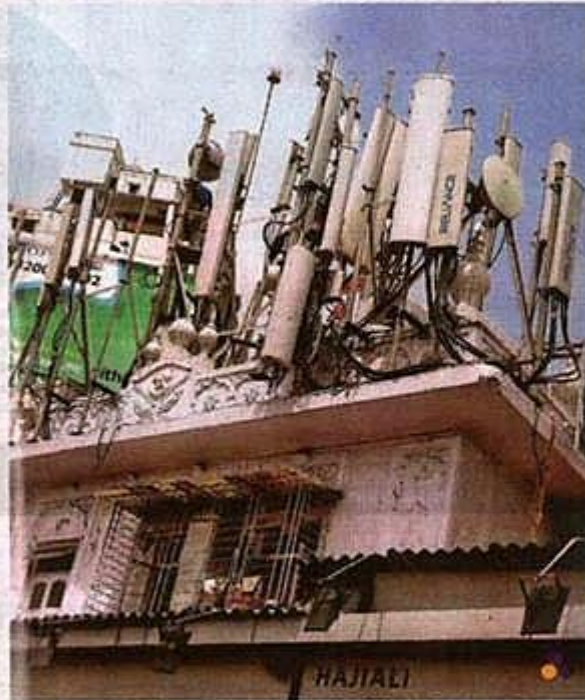
Multiple mobile phone antennae above Haji Ali Juice Centre
